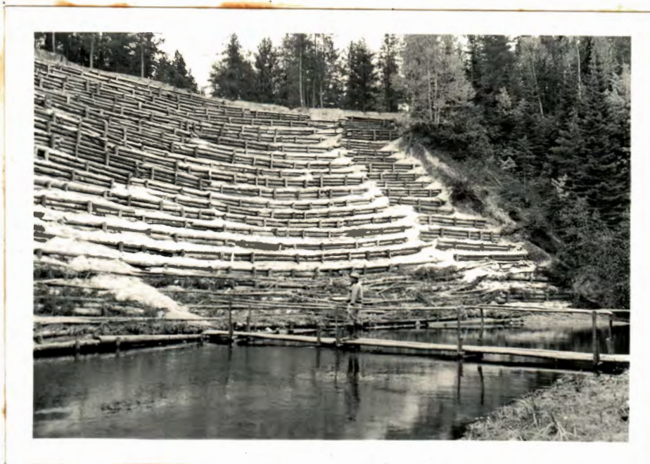
Recently completed erosion control work on Two Hearted River. Note tendency of sand to level off terraces.
