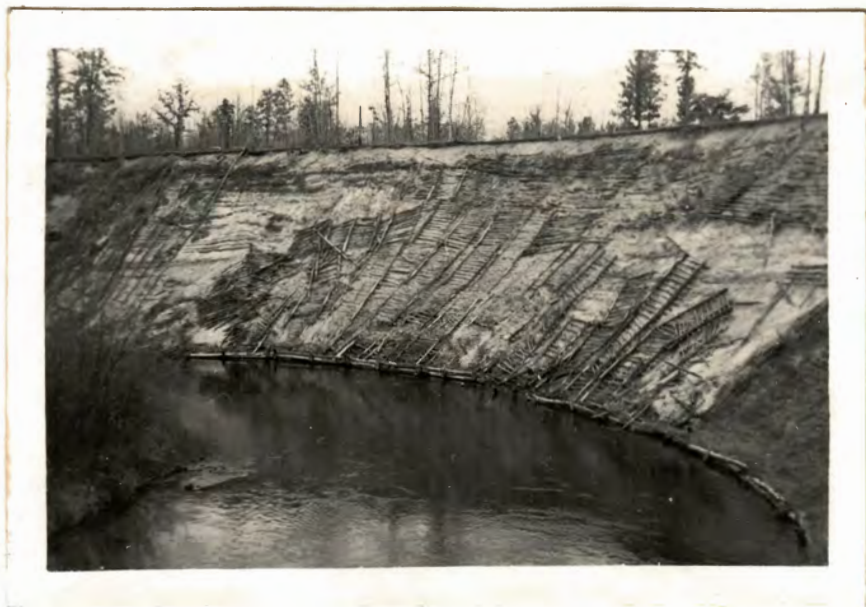
Erosion control work on Pere Marquette River just below mouth of Kinne Creek. Note points where sea-wall is broken. Age of work at time of photographing about four years.
