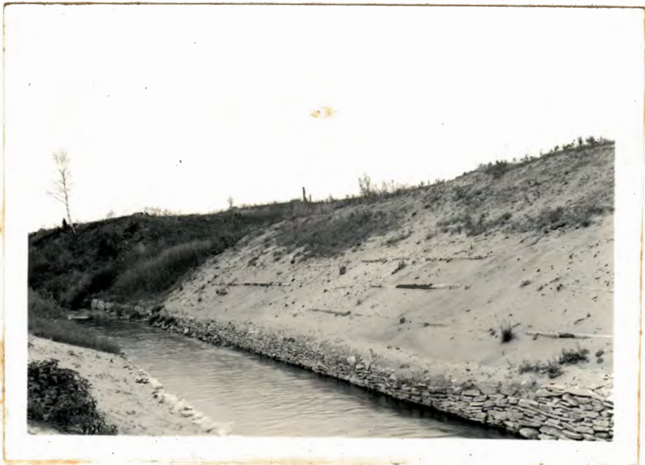
Erosion control along raceway, Fox River Rearing Station. Note stability of stone sea-wall, and establishment of vegetation on sand slope which has filled log terraces to normal angle of repose.
