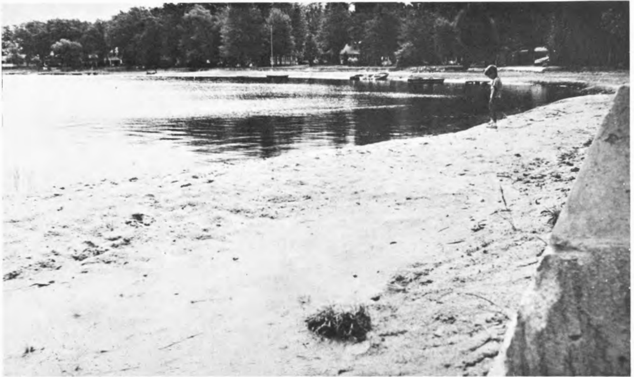
Scene 3: Sand beaches lay below the shoreline muck. The dredge and the bulldozers working as a team removed the muck creating clean sand beaches and deep clear water as they progressed.
