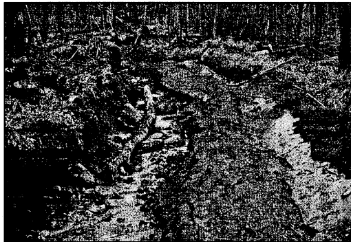
Figure 1. Forest Road Rutting Damage
